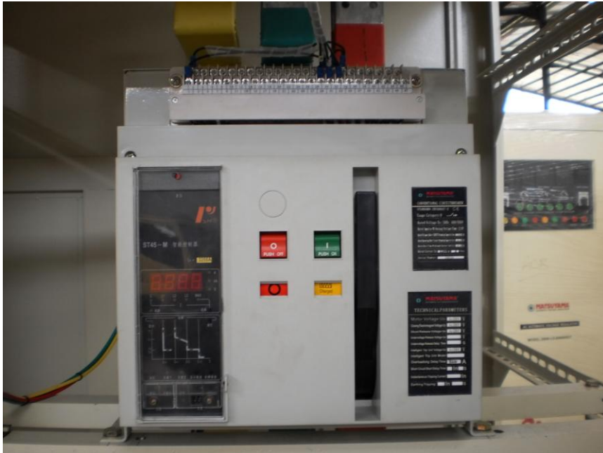
ACB (Breaker ON – OFF).
