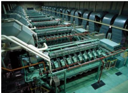
KU installed in Pakistan
