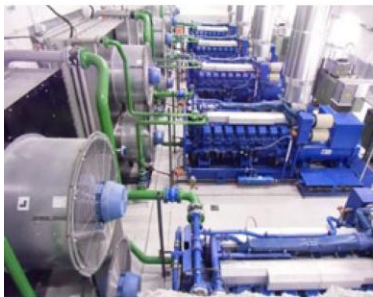
S16R installed in Amiens Hospital, France
